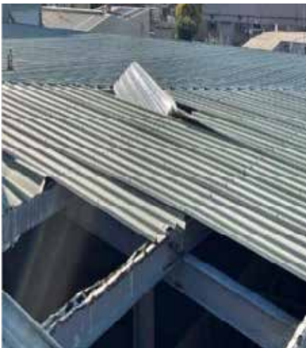
Storm damage October 2021
